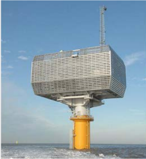
Figure 3. Offshore Power Substation. Source: https://www.jandenul.com/en/activities/offshore-services/offshore-wind-farms
